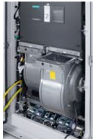
Replacing one of the two converter fans while the system is operational
